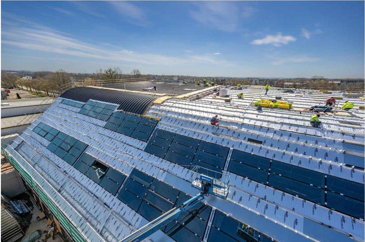
Long planning periods within corporations are normal. Rapid construction progress through motivated teamwork is BORA.
